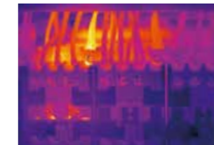
Maintaining plants: Identify excessively high temperatures in circuit breakers and electrical components before breakdowns can occur.
