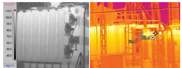
Normal transformer IR pattern
