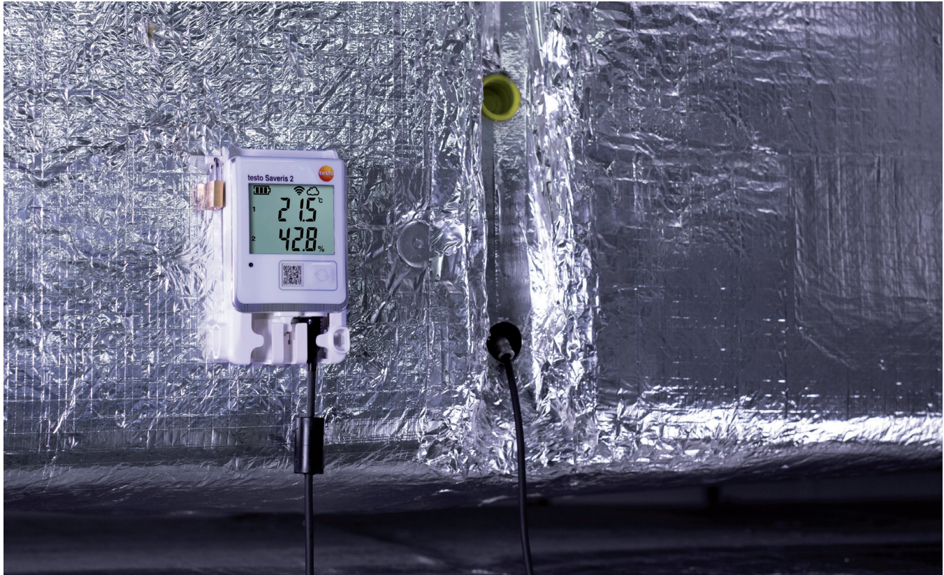
A testo Saveris 2 WiFi probe measures temperature and humidity in a ventilation duct.
