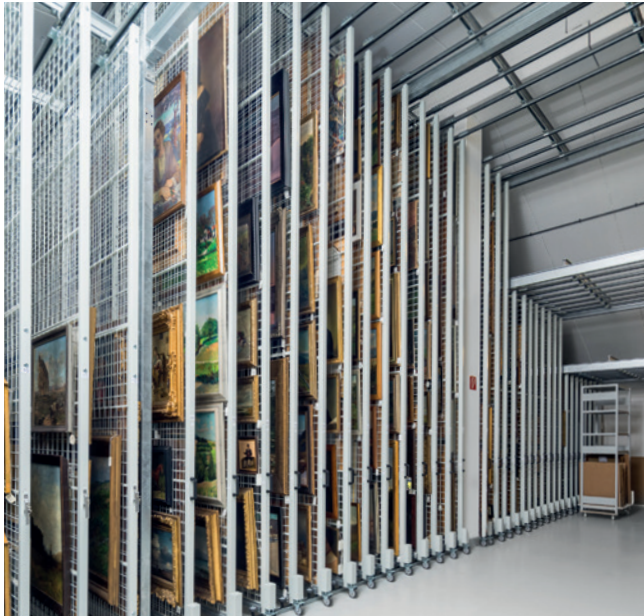
Measuring point for humidity and temperature in a depot.
