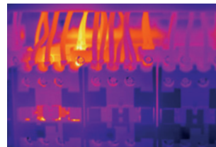
Maintaining plants: Identify excessively high temperatures in circuit breakers and electrical components before breakdowns can occur.
