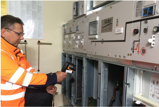
Figure 1: Thermographic measurement on a medium voltage switchgear.
