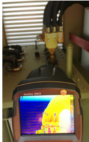
Figure 2: Thermographic image of the connection of a transformer (20,000 volts to 400 volts) via low-voltage cable.
