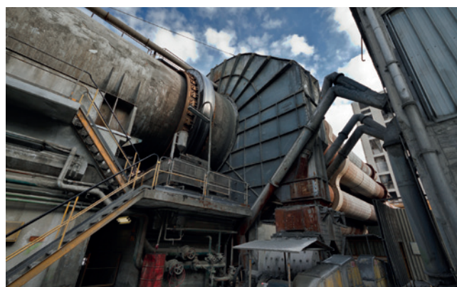
Firing the raw granulate in the pre-heating plant and the rotary kiln.
