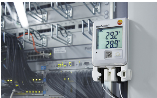
One system for all server rooms – even in different buildings.
