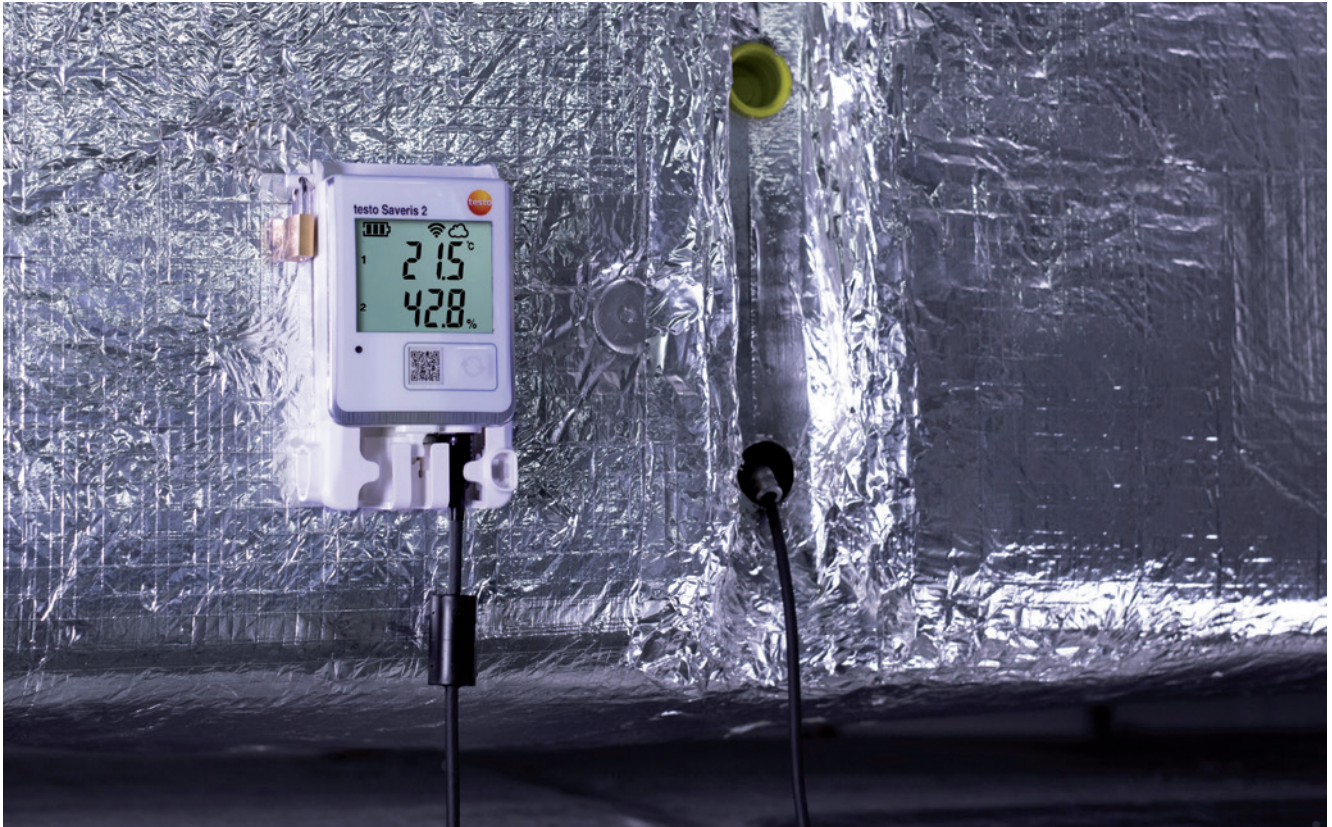
A testo Saveris 2 WiFi probe measures temperature and humidity in a ventilation duct.
