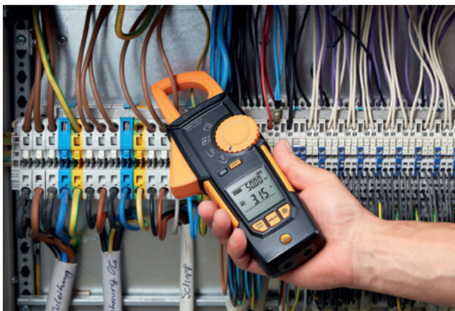
Measuring current in a switching cabinet.
