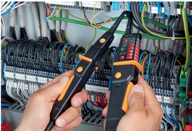
Measuring voltage in a switching cabinet.
