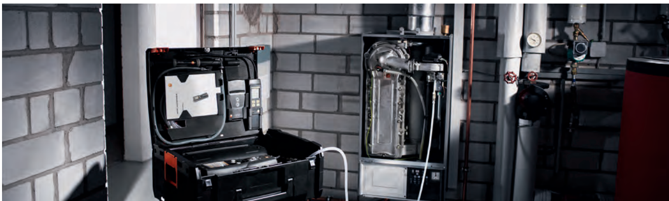
Automatic servicability test with gas-feed appliance with connection to the gas boiler
