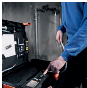
Automatic tightness test
